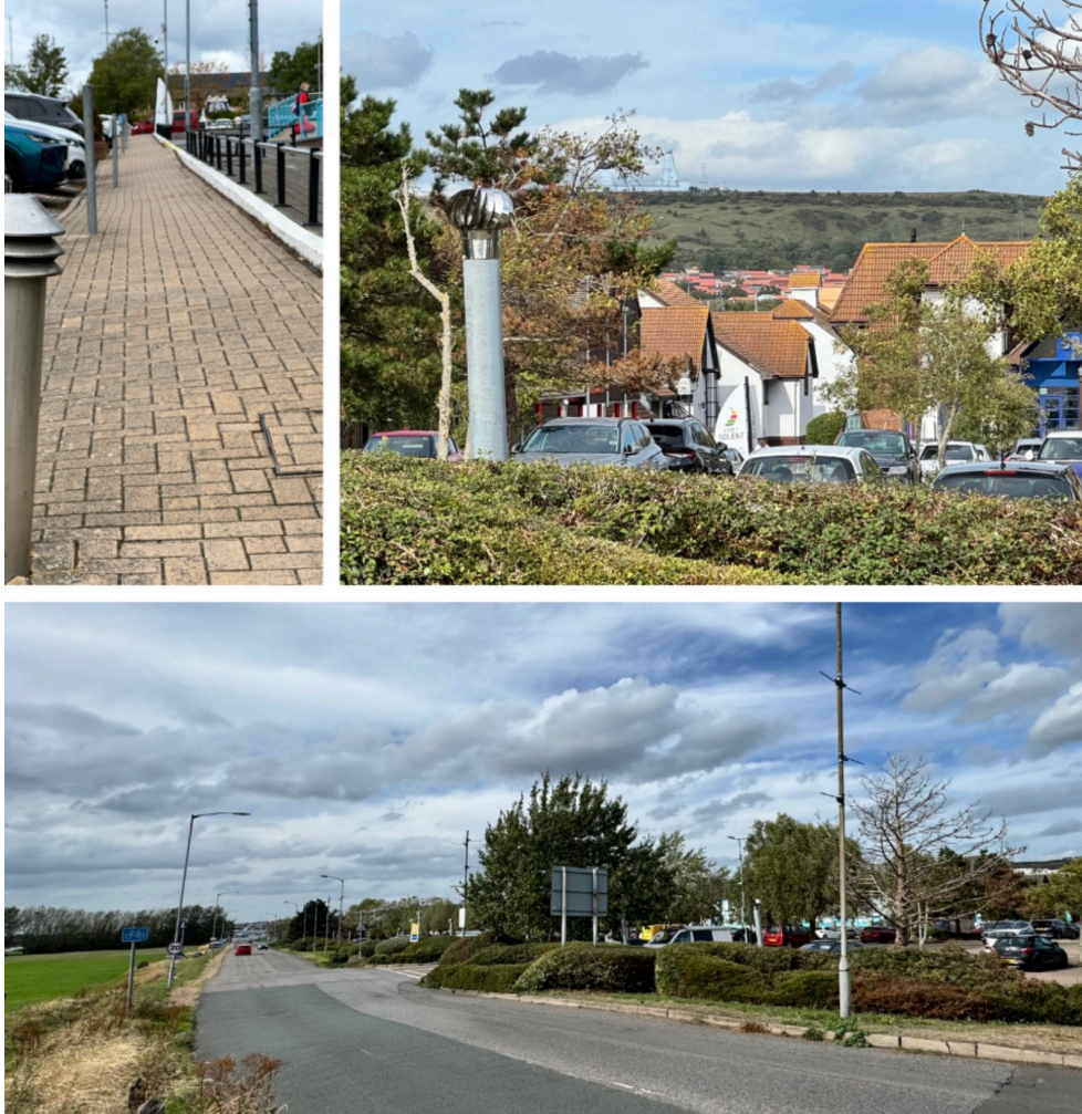
Photos taken September 2026: top left, outside David Lloyd gym showing lateral subsidence of the pathway and the same at the edge of the car park; top right, gas vent at edge of car park opposite the cinema where the proposed tall buildings will be concentrated and erected on ground that is already at a higher elevation than the rest of the marina thereby dominating the surroundings; bottom, Marina Keep showing buckling of the road surface due to ground movement.
